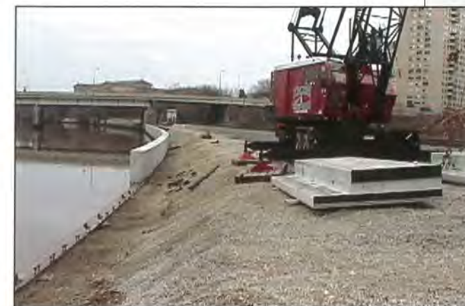
Crane installing pre-cast concrete panels at Cherry Street as part of the bulkhead project
